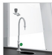
Water & Gas Tap Water Sink
